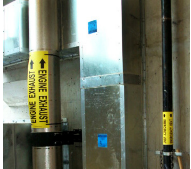
A fire-rated pipe enclosure.
